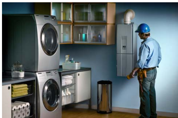
Tankless water heaters not only lower household energy bills but also save customers precious space.
